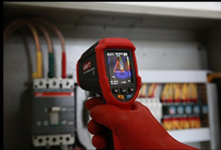
Power distribution cabinet inspection
